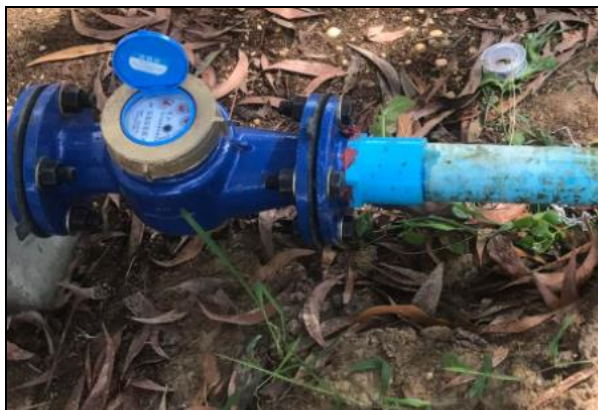
Figure 4.22: Water meter installed in the process water line
